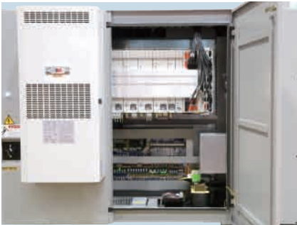
A/C Cooling System
